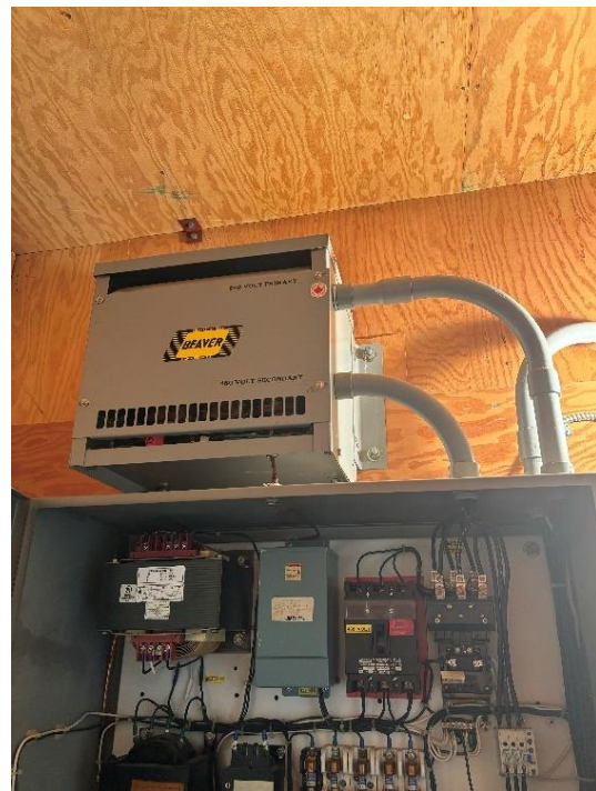
Figure 8 South Well House Electrical
