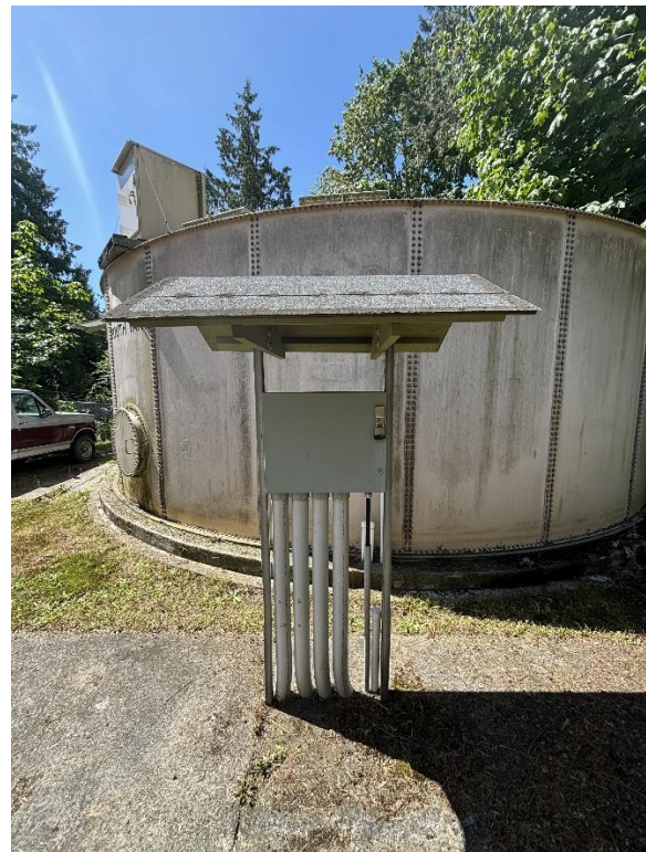
Figure 24 Future Electrical Expansion
