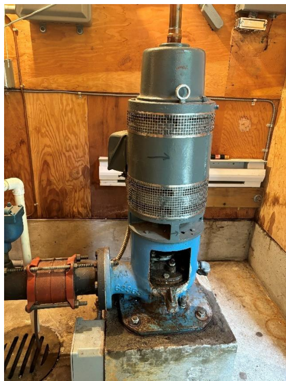
Figure 12 South Well House Pump
