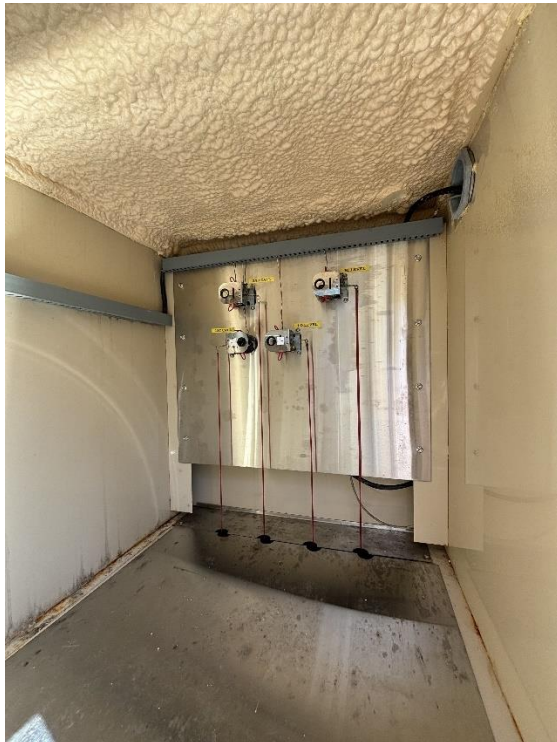
Figure 19 North Tank Float Controls
