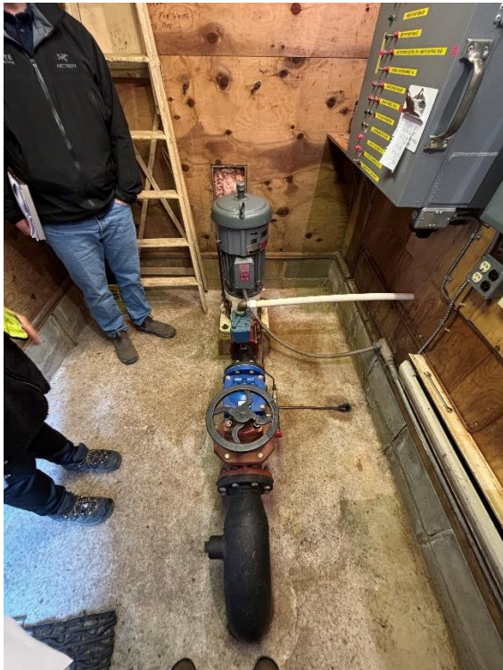
Figure 3 North Well House Piping Configuration
