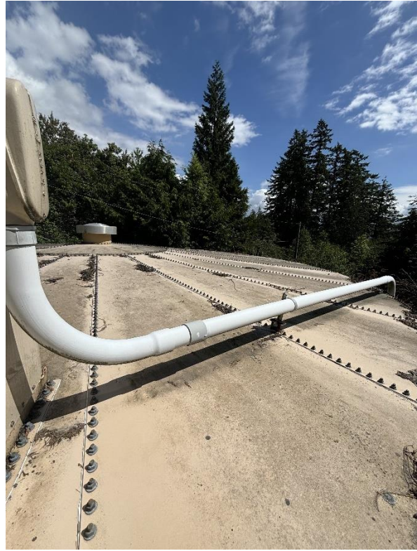
Figure 18 North Tank Flat Levels Electrical
