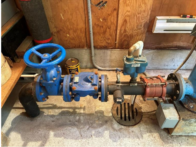
Figure 9 South Well House Piping
