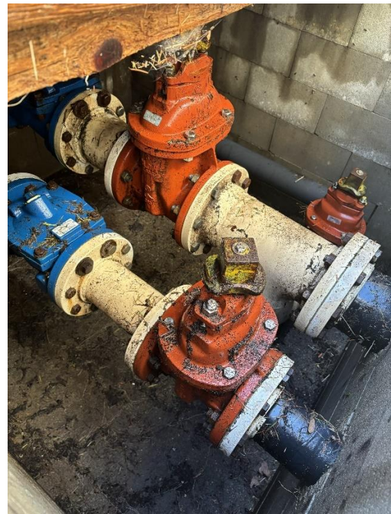
Figure 20 North Tank Valve Chamber
