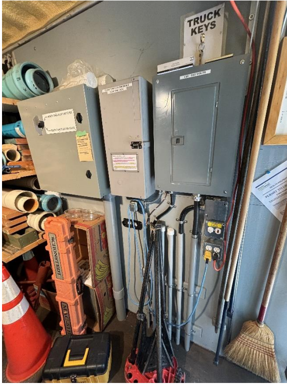
Figure 21 Site Electricals & Controls
