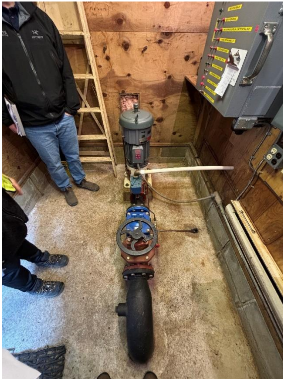
Figure 3 North Well House Piping Configuration
