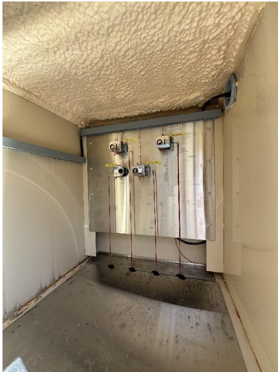
Figure 19 North Tank Float Controls
