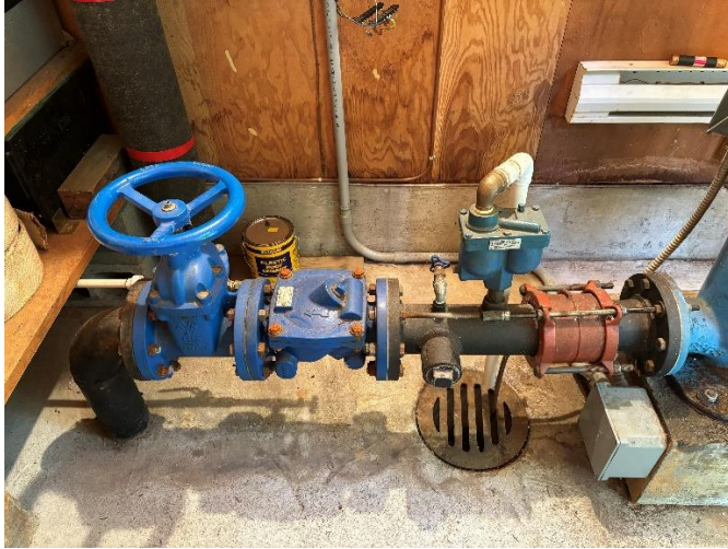
Figure 9 South Well House Piping
