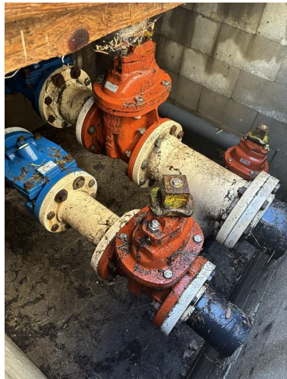
Figure 20 North Tank Valve Chamber
