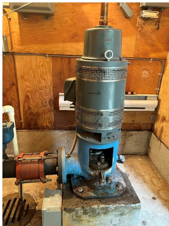
Figure 12 South Well House Pump
