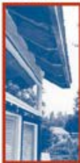
Open eaves, vents not screened (6 pts)
