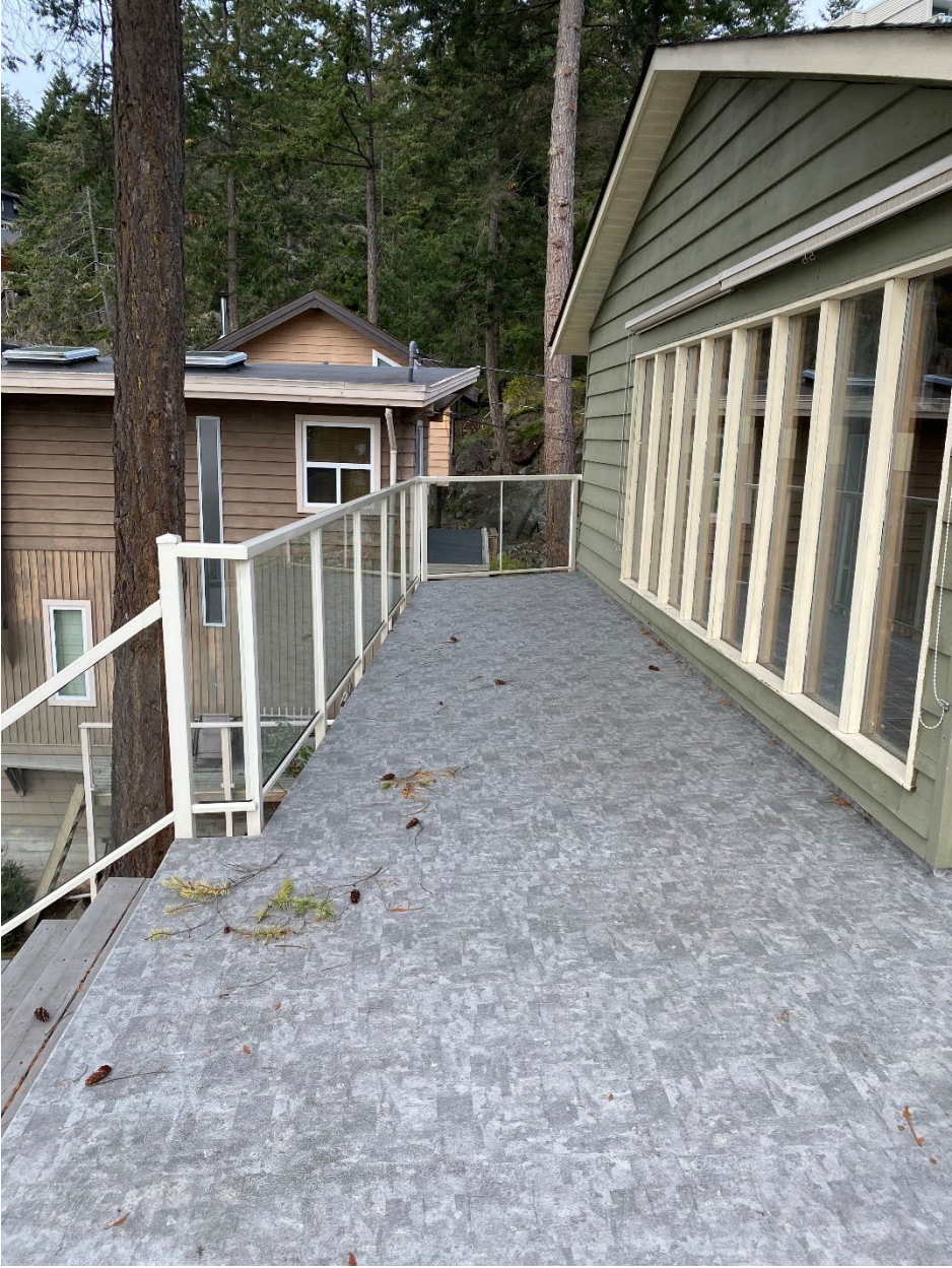
Figure 2: Upper deck to be replaced
