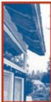
Open eaves, vents not screened (6 pts)
